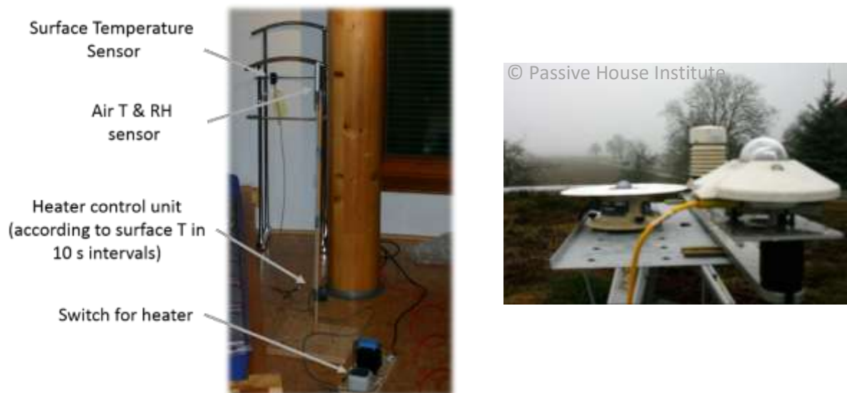
Figure 3 Decentralized control unit with sensors and switch for heater (left). Weather station on the roof of the building, with view on the surroundings.
